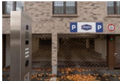
Garage access: D21x tower with door intercom system incl. RFID and Vingcard reader
